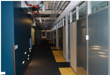
Below: A corridor with multiple TWXW sensors visible.
