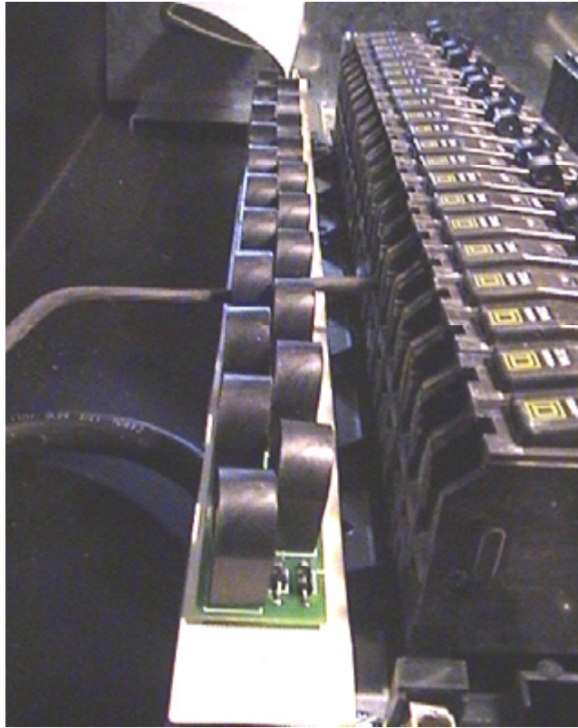
Figure 3 – CTs installed in a panelboard for branch circuit monitoring
